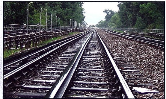
Restrictions: Chigwell-Roding Valley before works began when there were several temporary speed restrictions in place
